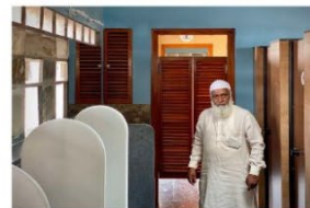
The slanted wooden doors allow flow of Light, Air & maintains privacy for the interior
