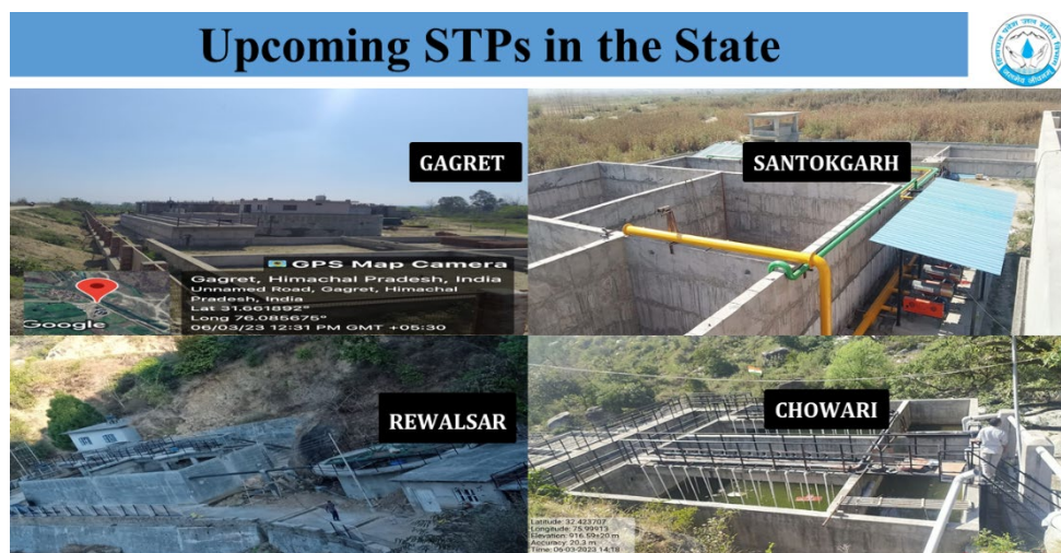
Figure 46: Completed and upcoming STPs of Himachal Pradesh
